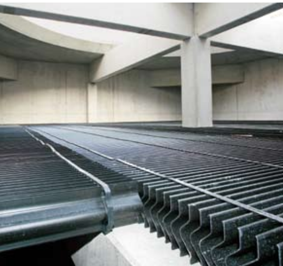
The combined gas and steam turbine power plant in Timelkam, Austria with a four-cell cooling tower.
